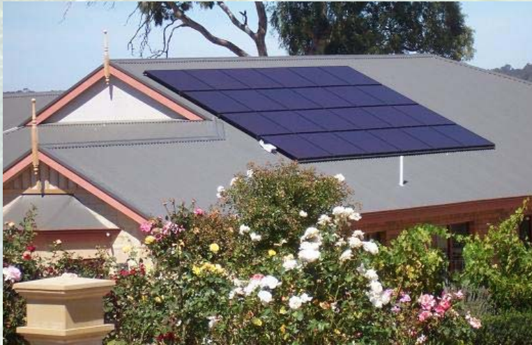
24 Kaneka thin film solar panels giving 1.4kW
