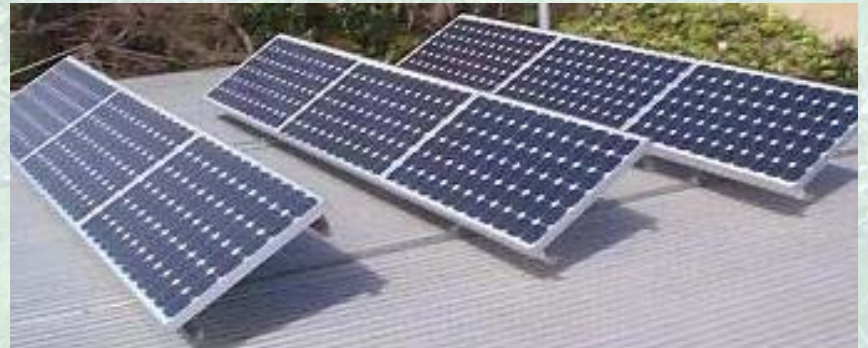
9 BP Solar mono-crystalline panels giving 1.6kW
