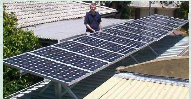
BP Solar mono-crystalline solar panels. 2,100W total
