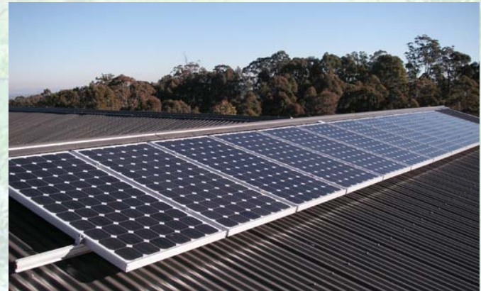
Solar panels - 2kW crystalline cells
