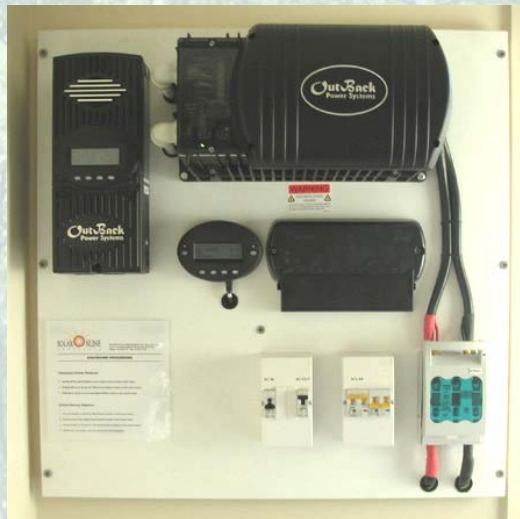
Inverter and battery charger
